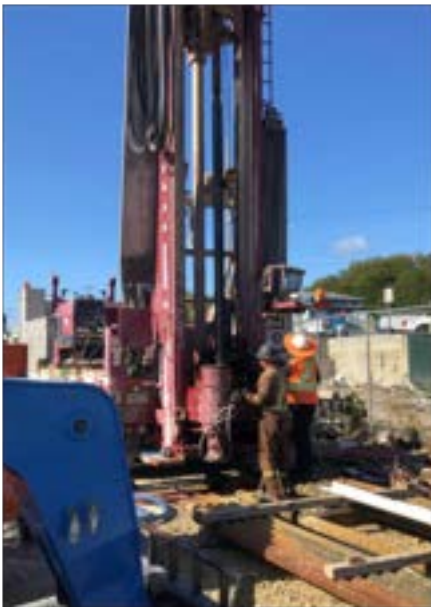
Drilling of test wells for hydrogeological study to use groundwater for cooling of the Energy Recovery Facility.
