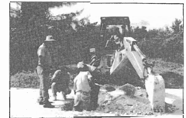
Water Authority operations staff complete a water service connection in Red Bay.
