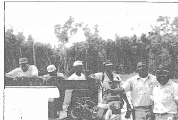
The New Works pipe line construction crew gets ready to start another day of work on a water main extension at the end of Hirst Road in Newlands
