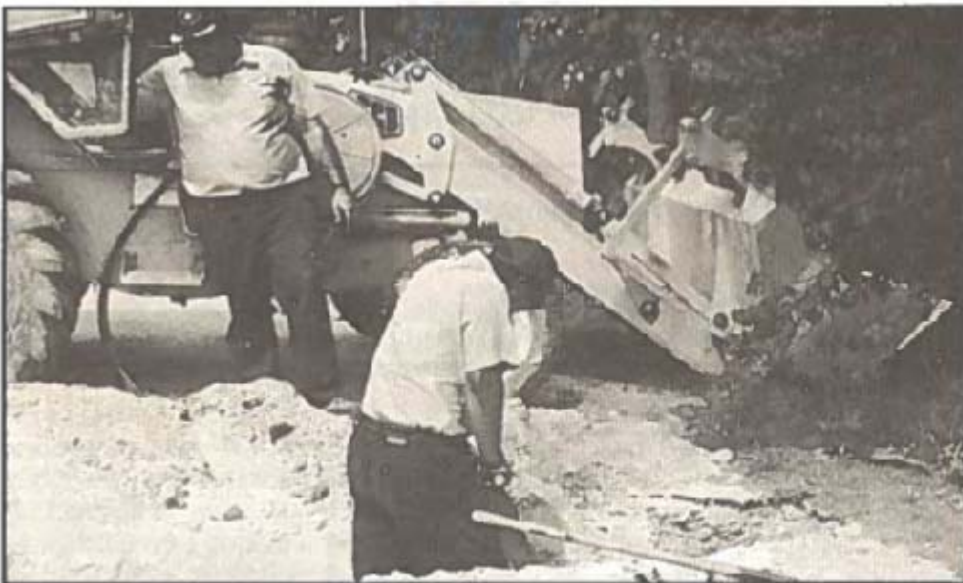
Brian Martinez, an Operator, using a hydraulic jack hammer to excavate a trench to lay a supply line across a road, whilst Walt Watler, the machine operator works the JCB excavator hydraulic controls.
