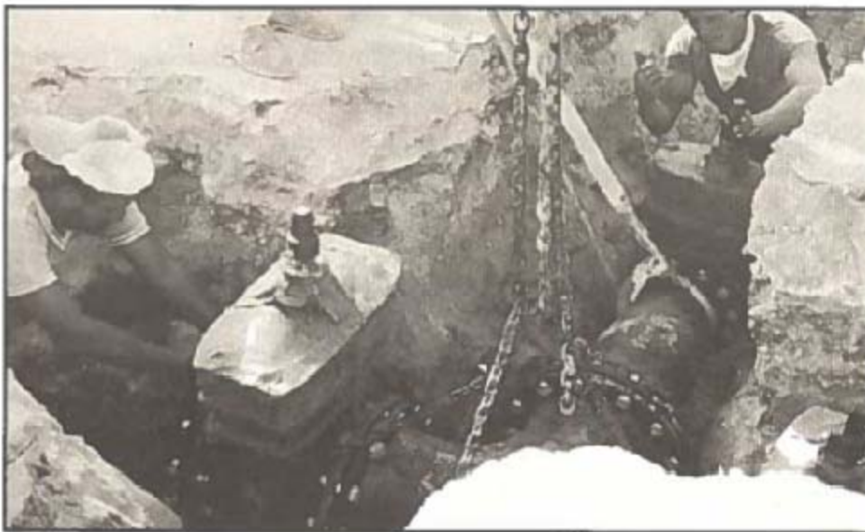
The water supply civil engineering contractor, Petroservicios, installing a valve system on the mainline in Savannah. Many such similar valving systems are incorporated in the distribution system so that individual areas can be isolated to allow repair or maintenance work without disturbing customers outside the area in which the work is being carried out.
